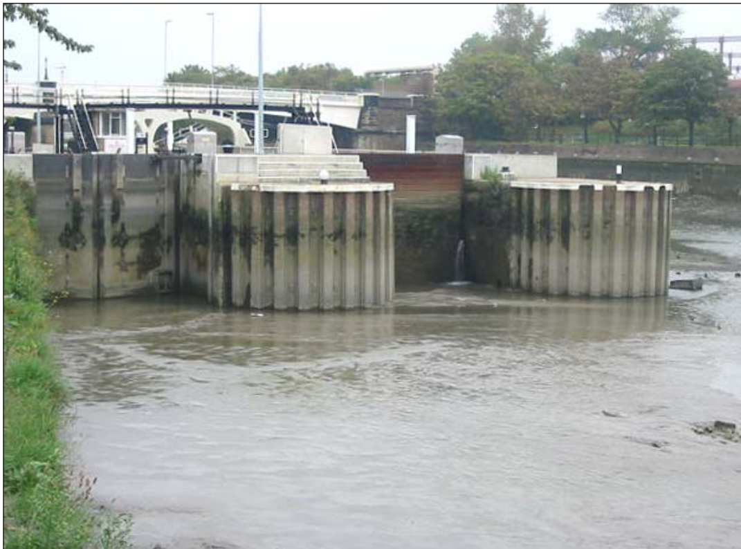
Bow Locks at low tide, and with the lack of use, a large mud bank is building up at the entrance.
