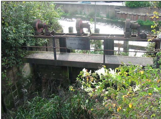
The overgrown sluice beside City Mill Lock. The lock is being reinstated and the sluice should also be brought back in service to restore the water management control.
